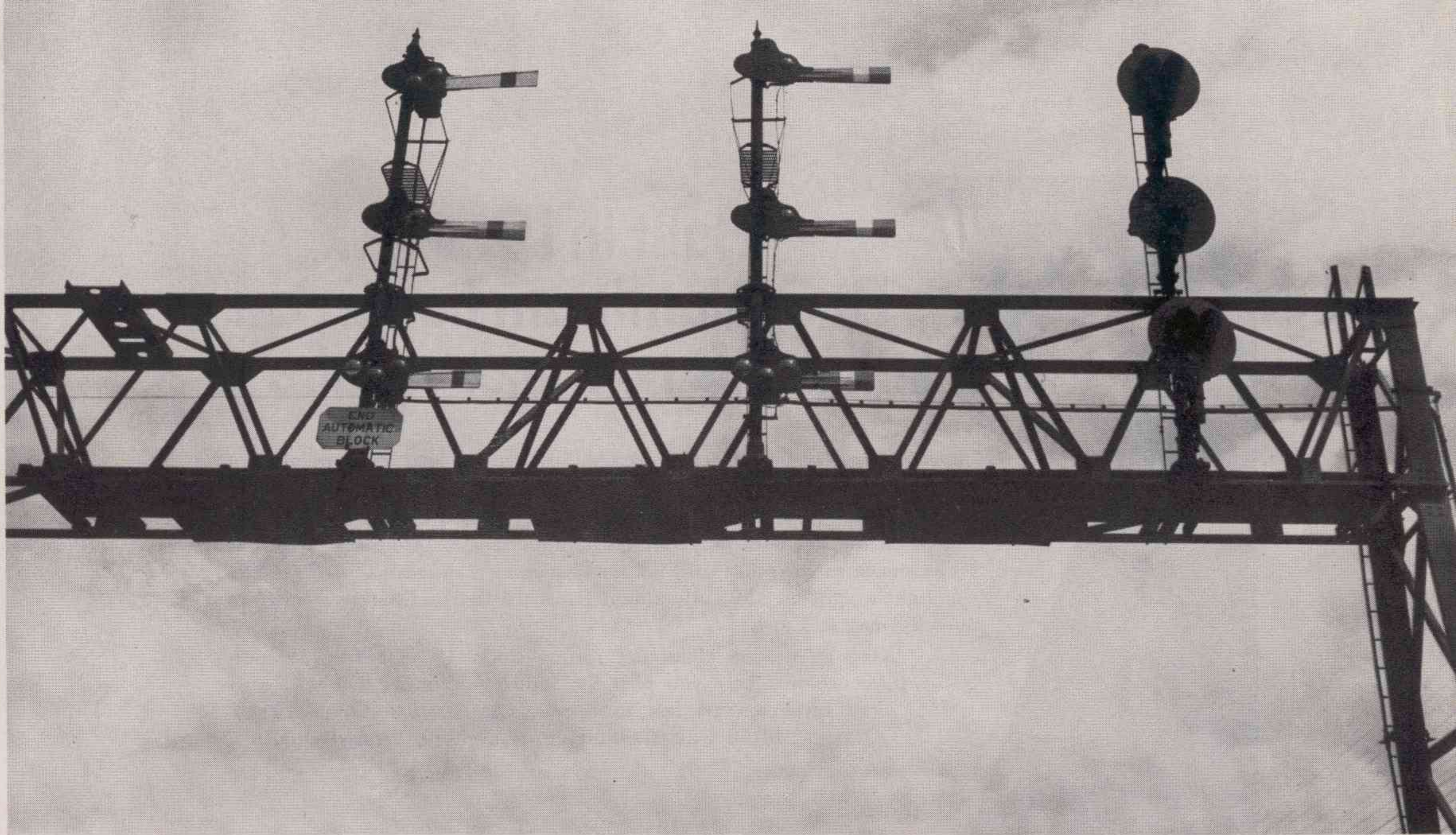
INTERLOCKER signals at Marion, Ohio. Although semaphore, color-light and position-light signals are in use, searchlight type is standard for new installations.
