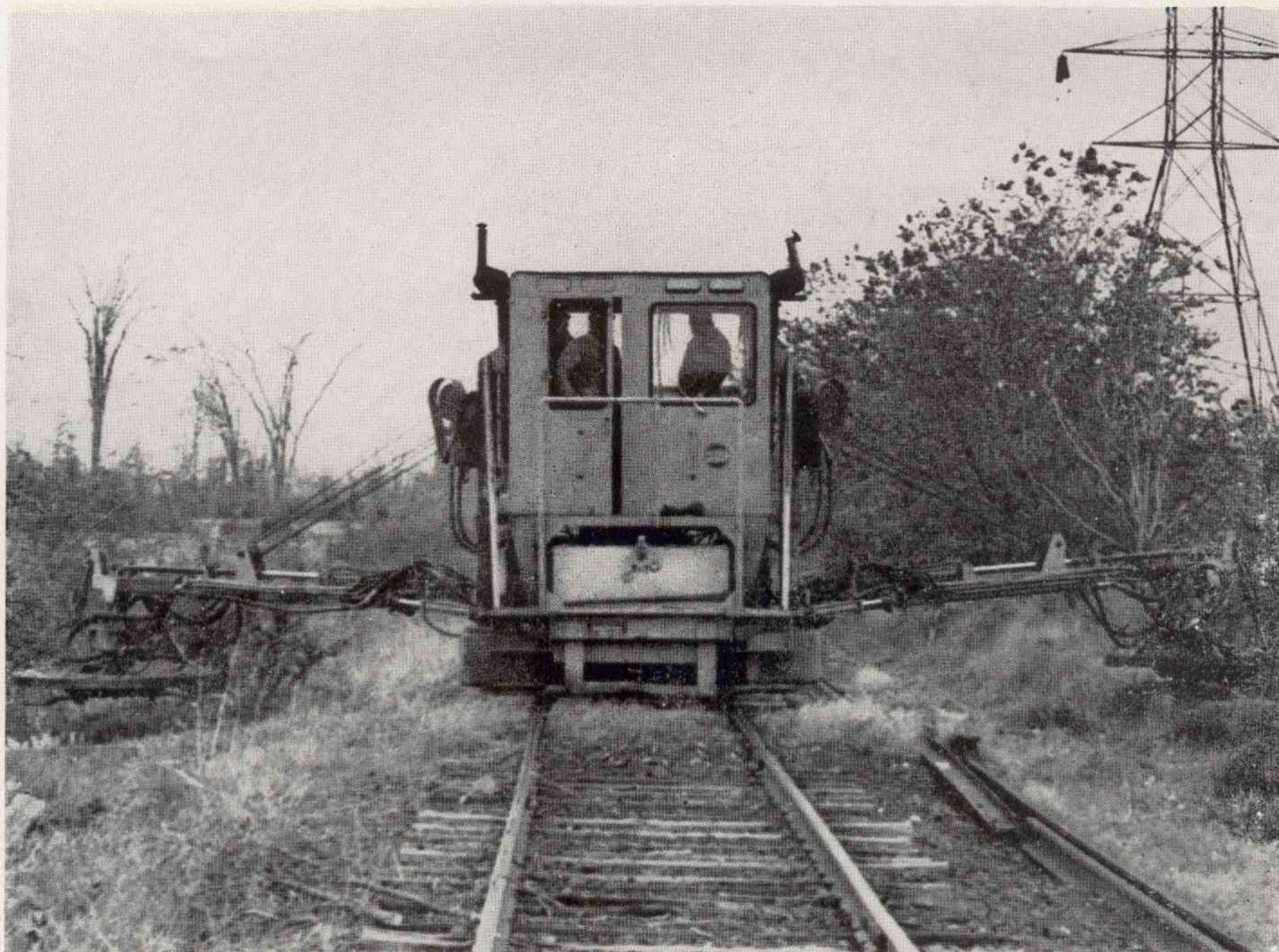
ON-TRACK brush cutter is used along lines where vegetation has grown up close to the track.
