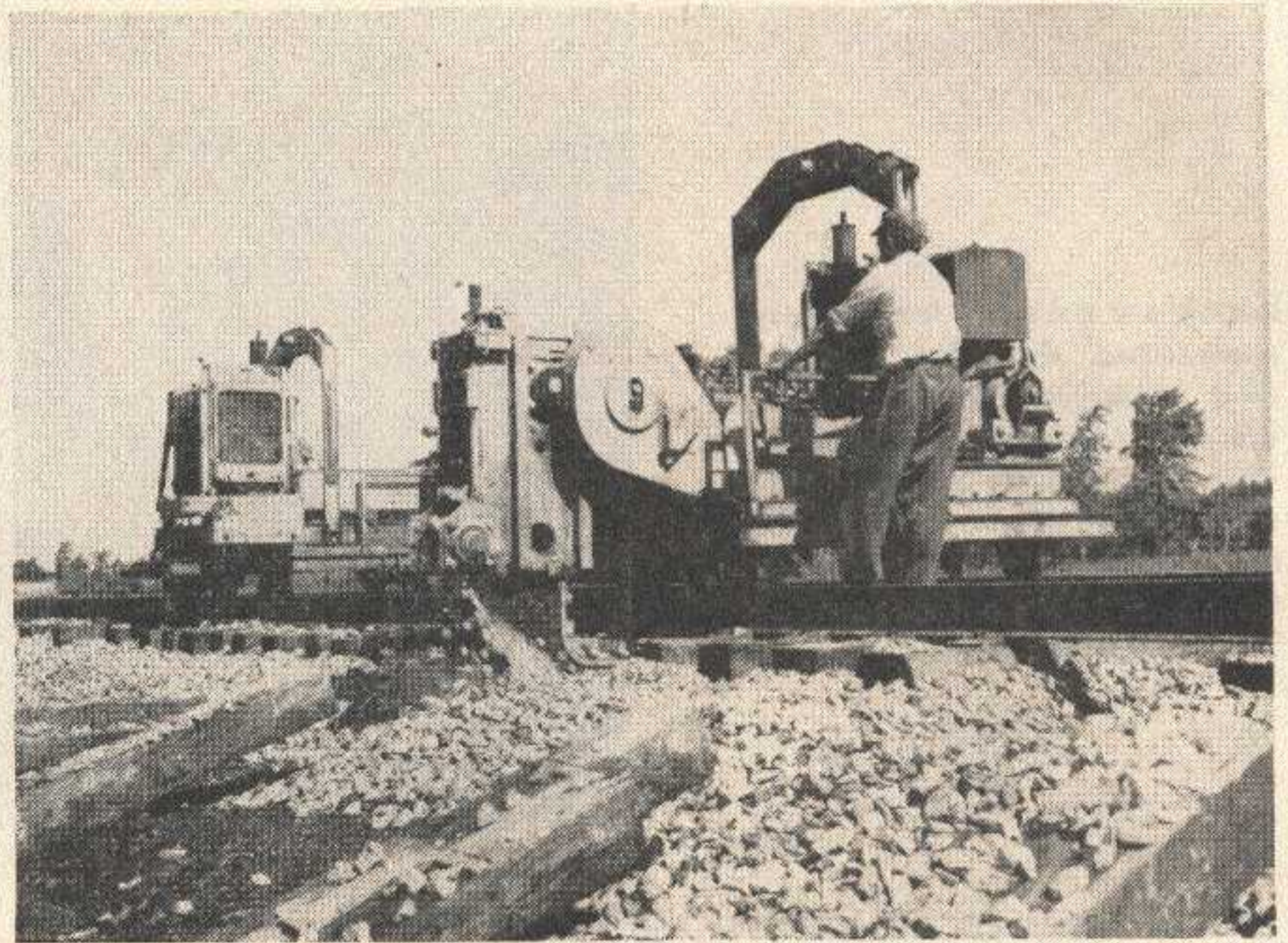
All out-of-face track maintenance operations are highly mechanized. This illustration shows two Cribex machines removing ballast from the track to facilitate the insertion of new ties
