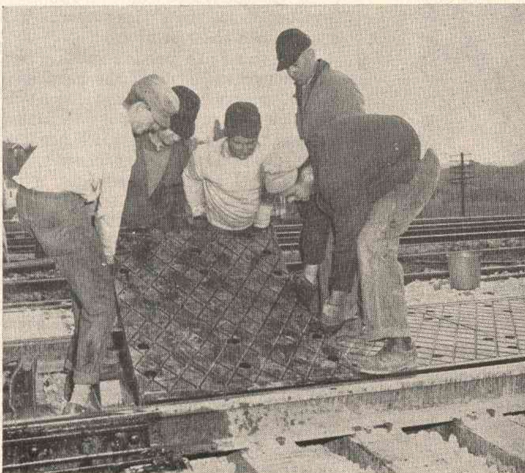
ONE END of slab for installation between the rails is placed against one rail after which the tapered . . .
