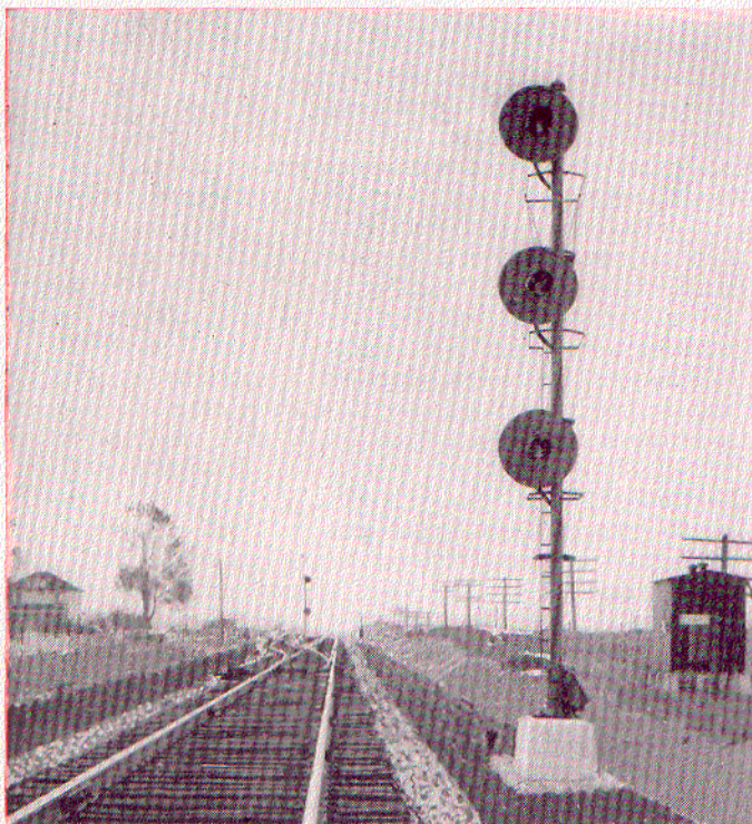
Signals and Power Switch At Johnsons
