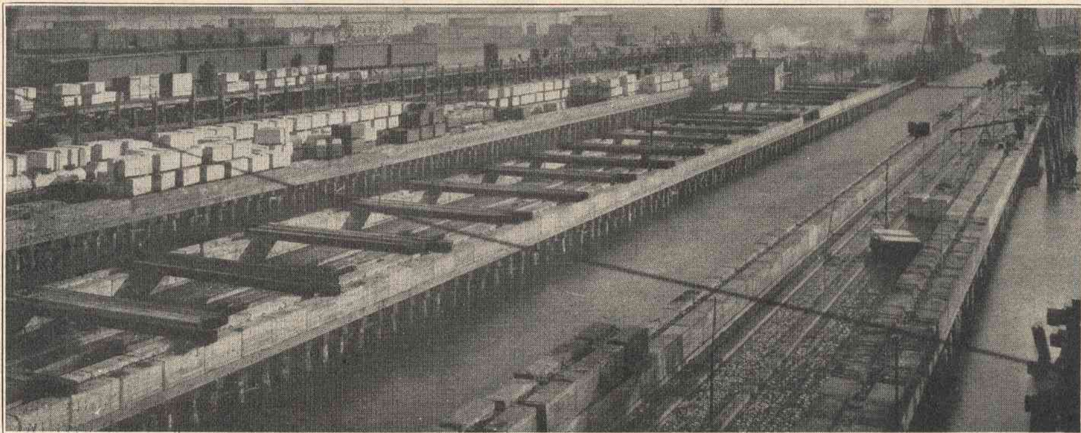
The Three Tiers of the Pier Sub-Structure at Various Stages of Construction. Note the Precast Concrete Blocks in Place Above the Piling
