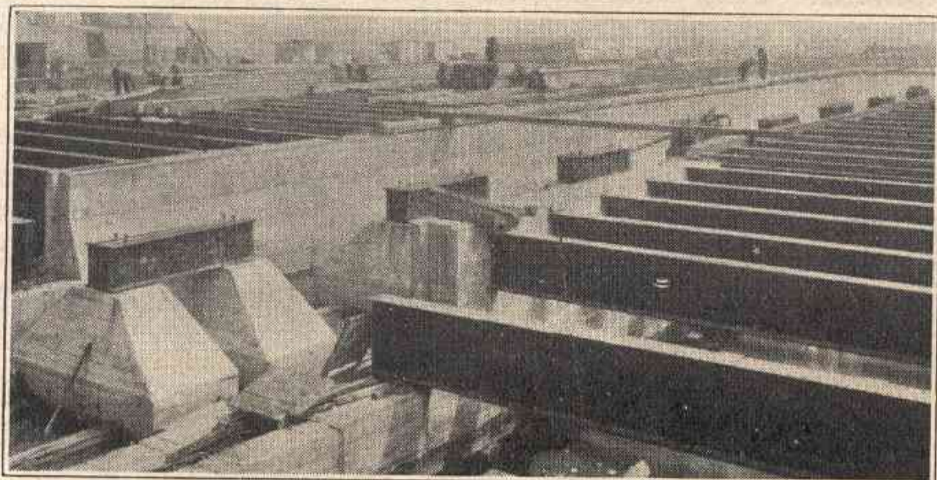
View Showing the Twin Concrete Pedestals for Supporting the Center Columns of the Pier, and the Heavy Structural Beams to Support the Floor System
