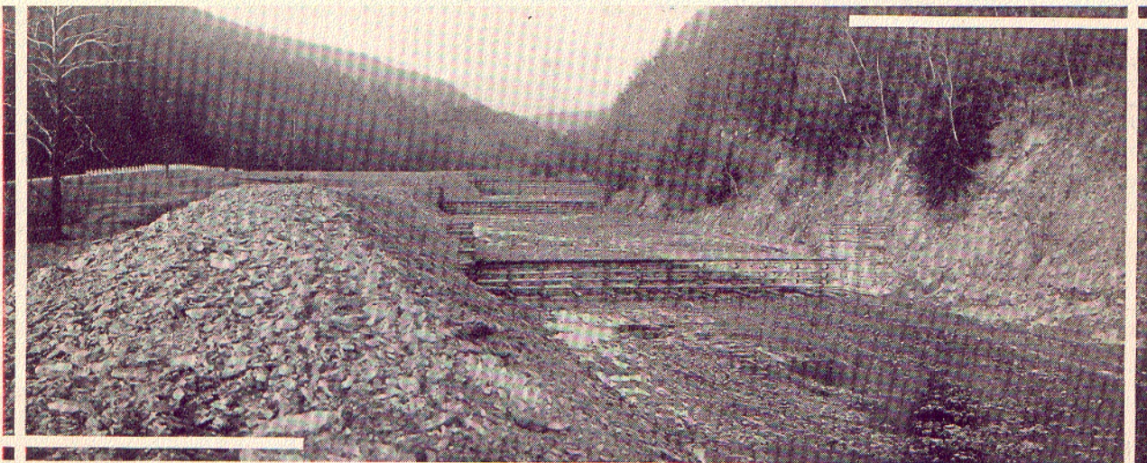
Seven Spillways Were Constructed in Stephens Creek to Produce A Non-Eroding Grade
