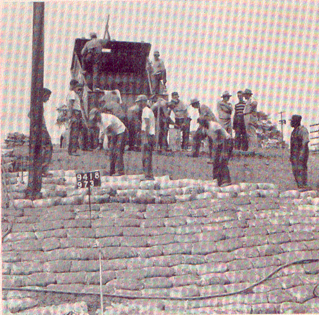
2 CONCRETE was delivered to the site in trucks equipped with special bodies designed to dump it into cement sacks . . .
