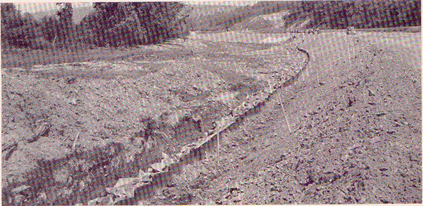
1 SHEETPILING was driven in accordance with the cross-section bagged riprap where it would normally be exposed to the direct flow of water. Elsewhere, rock-filled trenches sufficed (4) shown on the opposite page to anchor the toe of the
