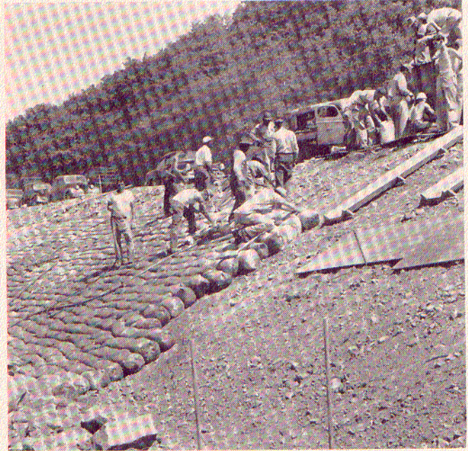
3 . . . FILLED BAGS, stapled shut, were allowed to slide on wood skids down the embankment; then set on edge and tamped
